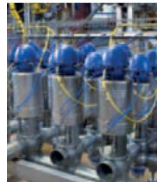
Complete flow battery at protein processing plant, Germany
